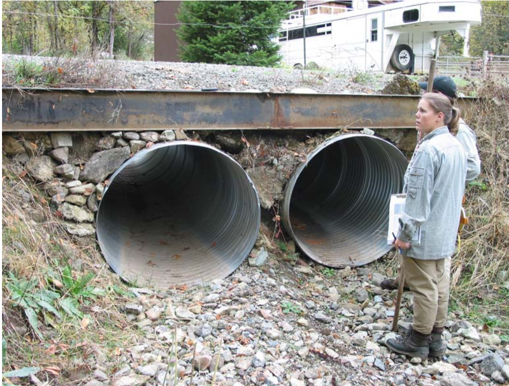
Figure 25. Culvert #3 outlet on Jordan Creek at driveway off Rod & Gun Club Road.
