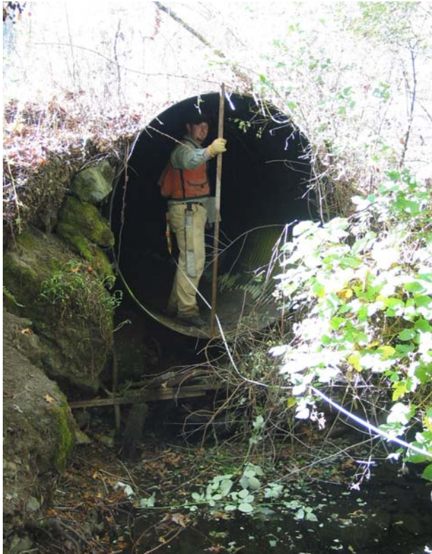
Figure 34. Culvert #11 outlet on Alder Creek at Canyonville-Riddle Road.
