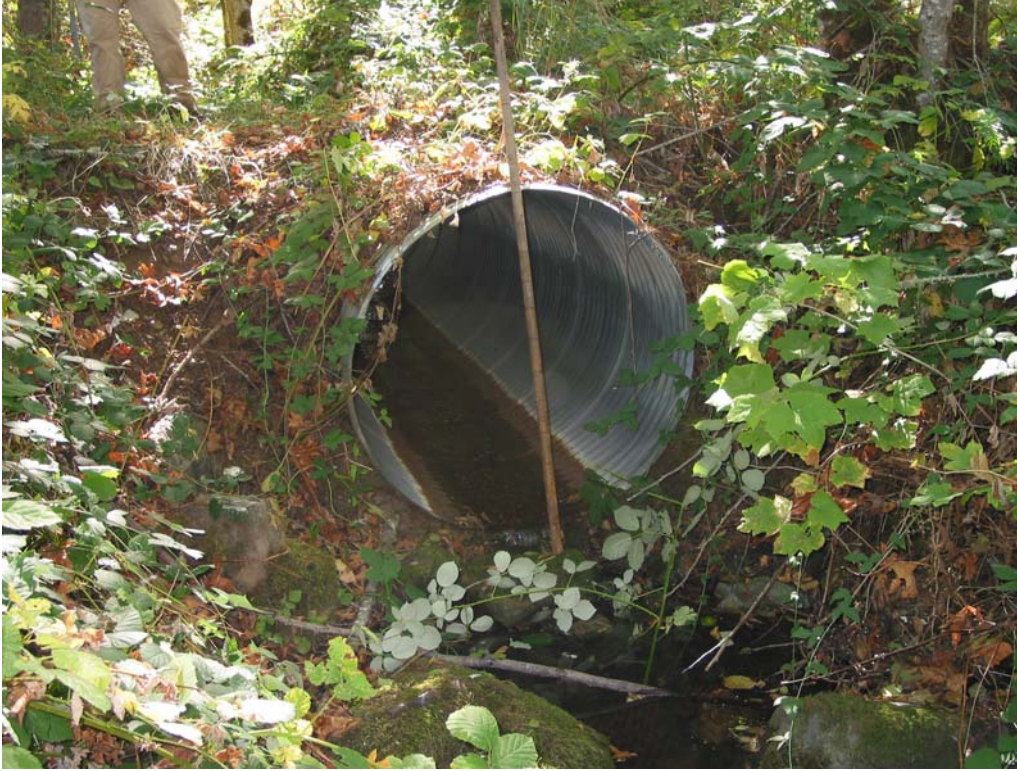
Figure 35. Culvert #12 outlet on Alder Creek at forest road south of Canyonville-Riddle Road.
