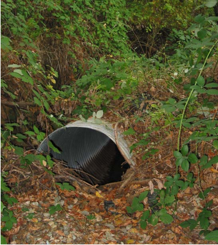
Figure 31. Culvert #8 inlet on Alder Creek at washed-out road off Meyer Lane.
