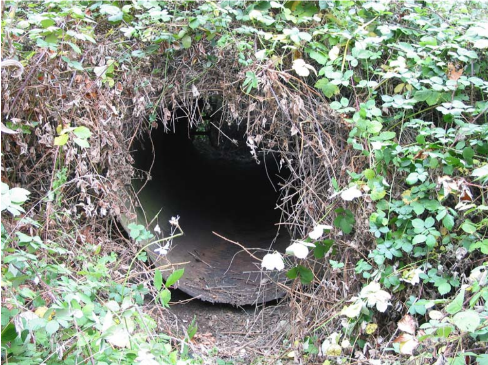
Figure 28. Culvert #6 outlet on Jordan Creek at south end of Rod & Gun Club Road.
